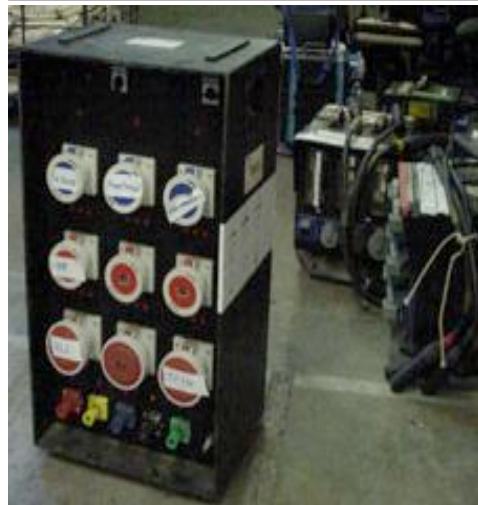
Photograph No. 8. Showing example of Distribution Unit with ‘Ceeform’ type outlet connectors, with Type 3 inlets to old colour scheme.
